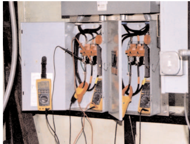
Simultaneous current and voltage logging at the control panel for two drive motors.
